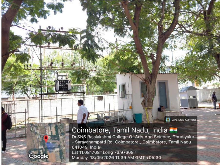
Power House – Transformer
