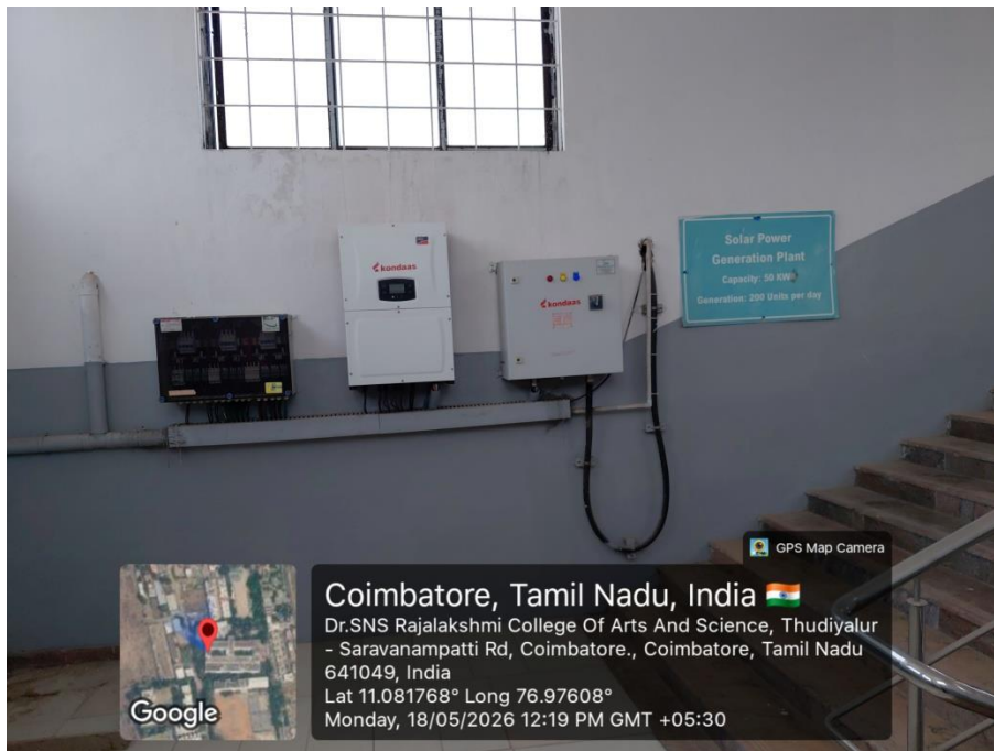
Solar Power Grid / Panels
